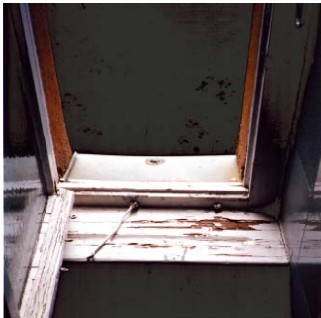
Leaky window - mold is beginning to rot the wooden frame and windowsill
